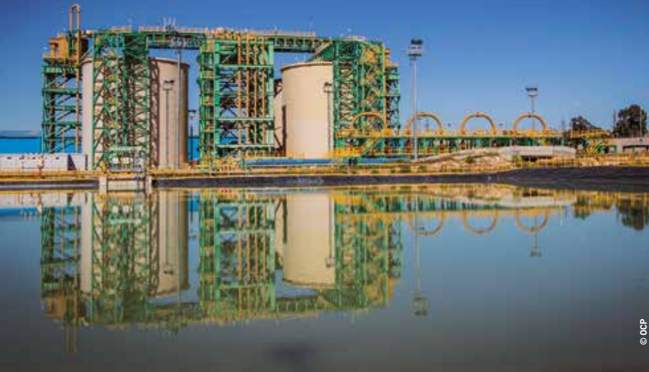
Station tête Slurry pipeline (OCP).
